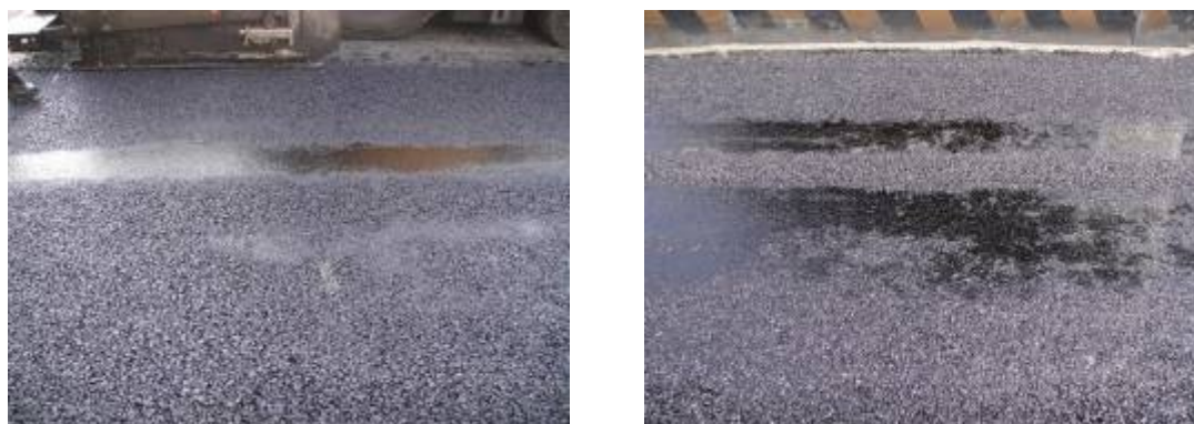
(a) BOF SMA 鋪面油斑 I
