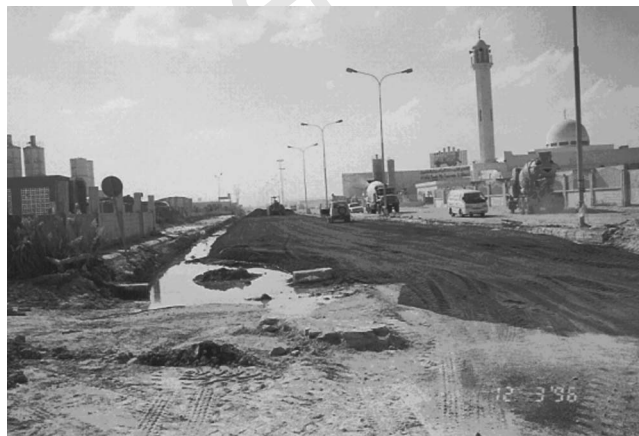
FIG. 12—A photograph demonstrating the construction of the road using SSA as a base course layer in an area with a shallow groundwater table.
